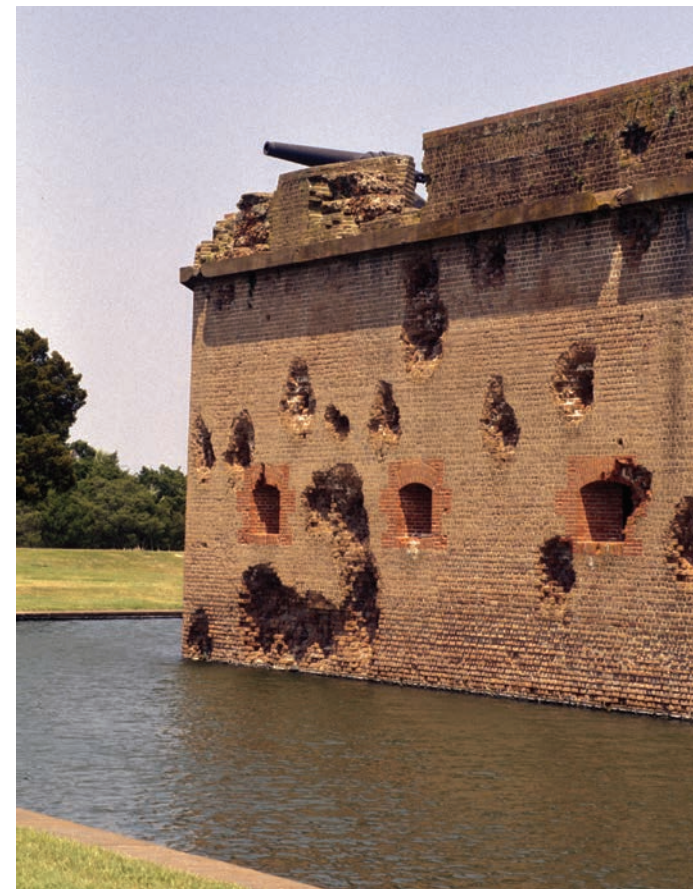
The thick walls of Fort Pulaski suffered extensive damage from Union artillery during the bombardment in April 1862.
